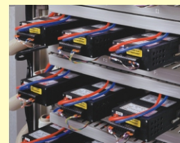
Rear of the panel door with the DPM50's fitted. All wiring and tubing is properly secured in cable trays. Designed for easy access during calibration in future.
